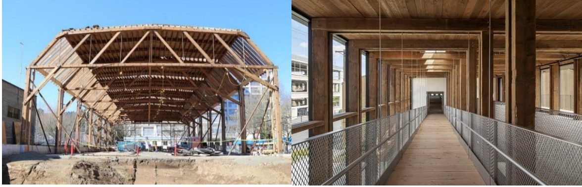
Abbildung 26 Redfox Commons alt (Portland) © Lever Architecture Abbildung 27 Redfox Commons neu (Portland) © Lever Architecture
